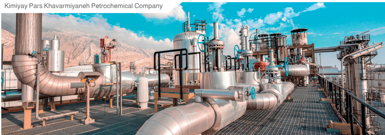
Kimiya Pars Khavarmiyaneh Petrochemical Company
